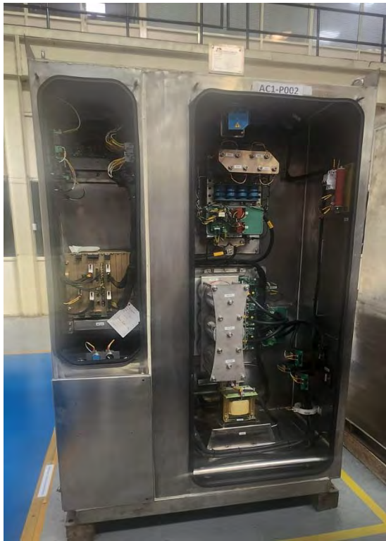
Auxiliary Converter (under assembling process)
