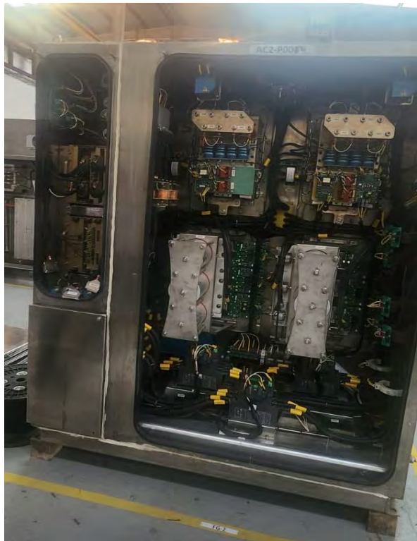
Auxiliary Converter (under assembling process)
