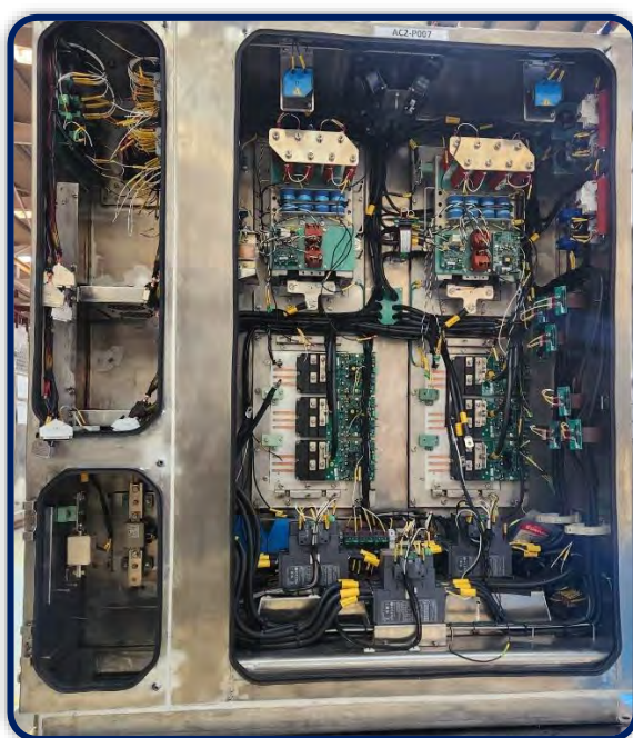
Inside view of Auxiliary converter
