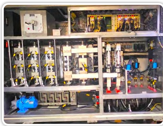
Inside view of Traction converter
